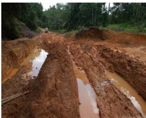
Plate 2: Showing a failed road in the study area Source: Authors field survey, 2017
