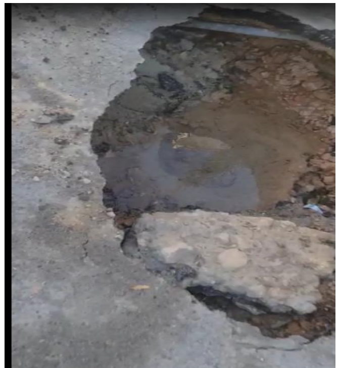
Fig. 8 Water leakage under the asphalt layer.
