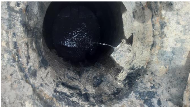
Fig. 4 Illegal connections on the main network in the city Of Ajdabiya.
