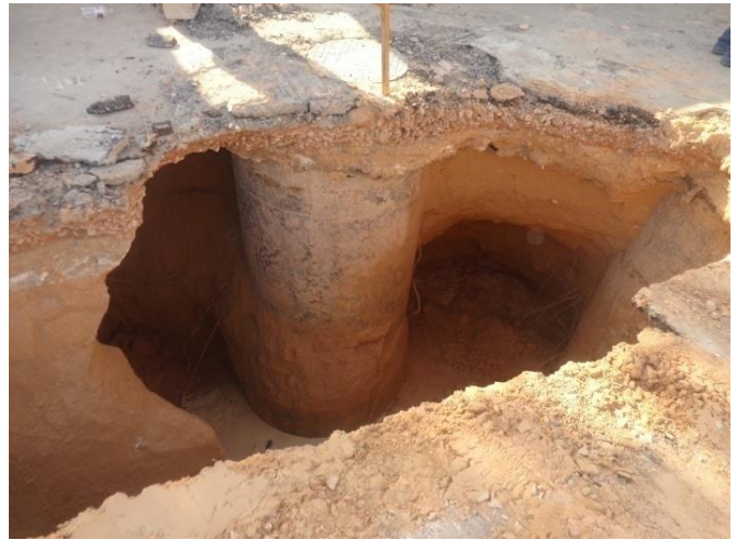
Fig. 10 Soil erosion due to leaks.
