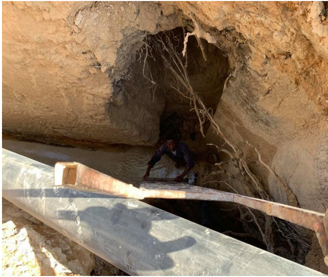
Fig. 6 Root trees and their effects on sewer network. 4.2 Effects of Underground Pipeline Leakage
