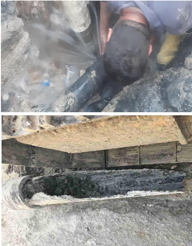
Fig. 3 Corrosion pipe in the city
