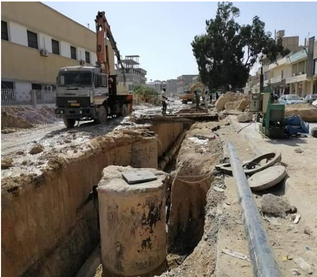
Fig. 1 Close-up of ruptured sewer rusty pipeline which causes sewage leakage stream and pollution. Old infrastructure issues in the city (Tripoli Street).
